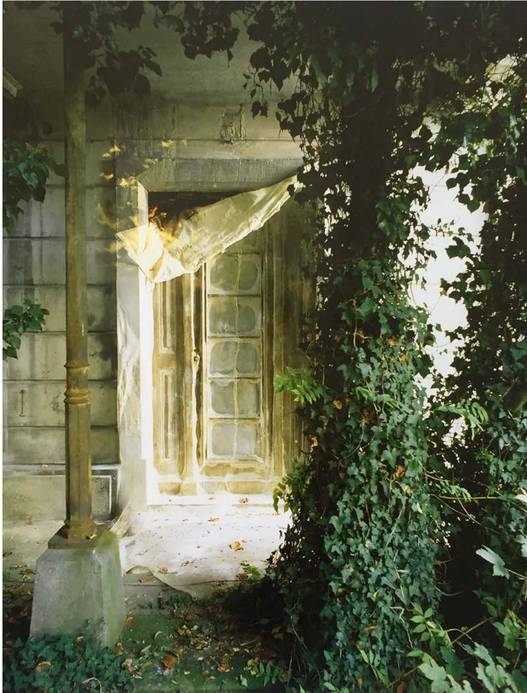
Skinning of the doors and windows at the abandoned Bellevue mental health institution, 1988
